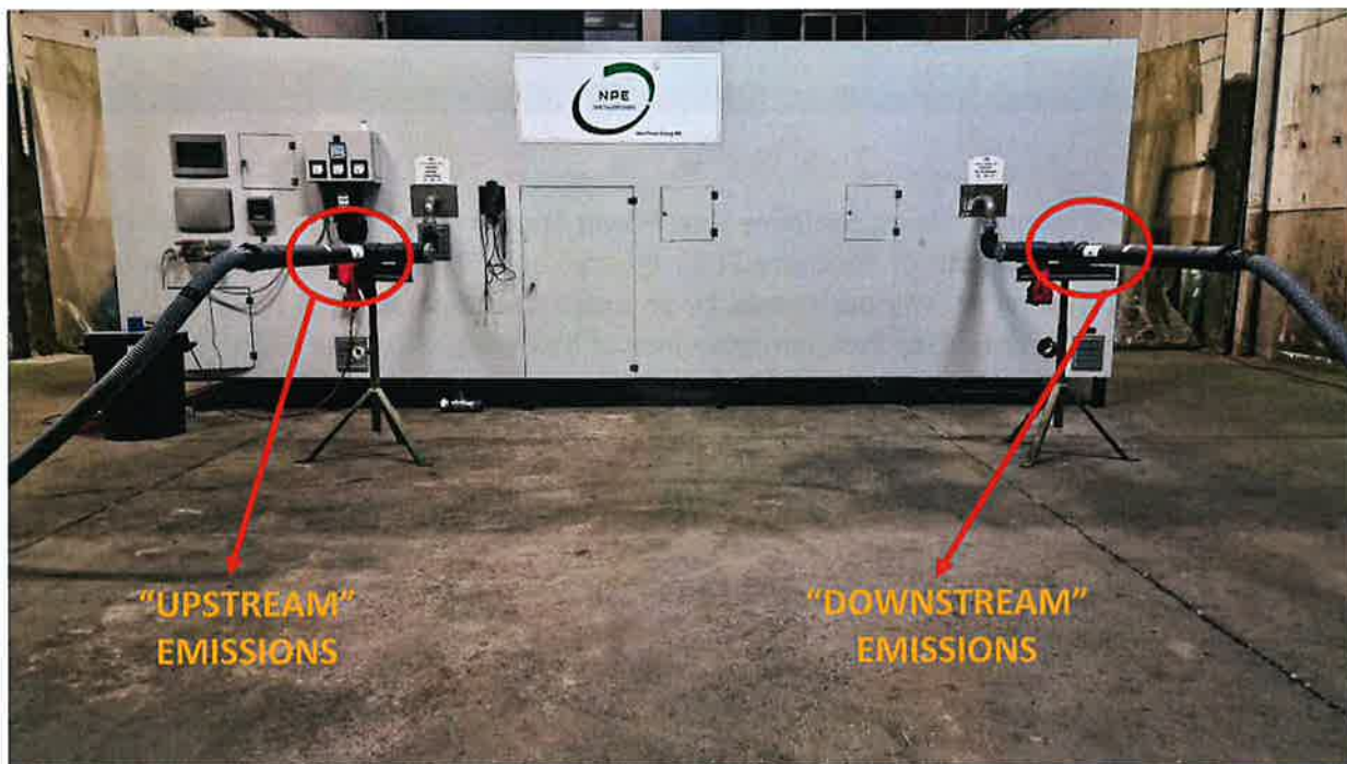
Fig. 2: External "Box" of the NPE air filtration system.
